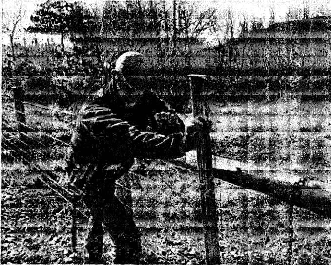
Fencing contractor Jake Wilson installs additional fencing on the Hoffman/Whitescarver property to keep their cattle out of the South Fork of the Shenandoah River.
